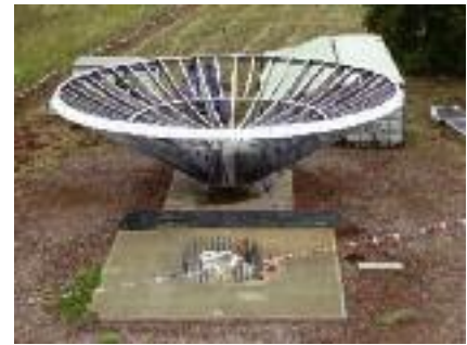
A 12-metre antenna is being built at Parkes to test equipment for ASKAP. The antenna itself is “off-the-shelf” from a commercial firm, and does not reflect what the final ASKAP antennae will look like.
